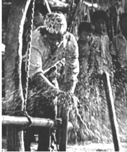
Figure 8.28: Man on scaffolding of drill at lowering drill fluid and cuttings to escape.
