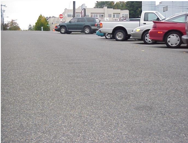
Corrugations on a street
