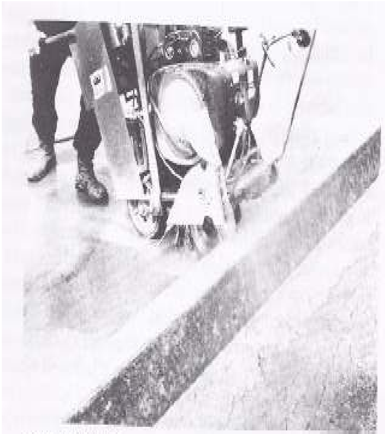
FIGURE 20-20 Concrete saw with a diamond blade cutting a pavement joint. (Courtesy Portland Cement Association.)
