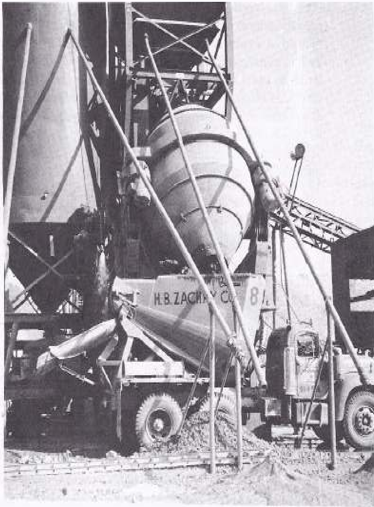
FIGURE 20-14 Tilting drum mixer discharging concrete into agitating body truck. (Courtesy Wire Reinforcement Institute.)
