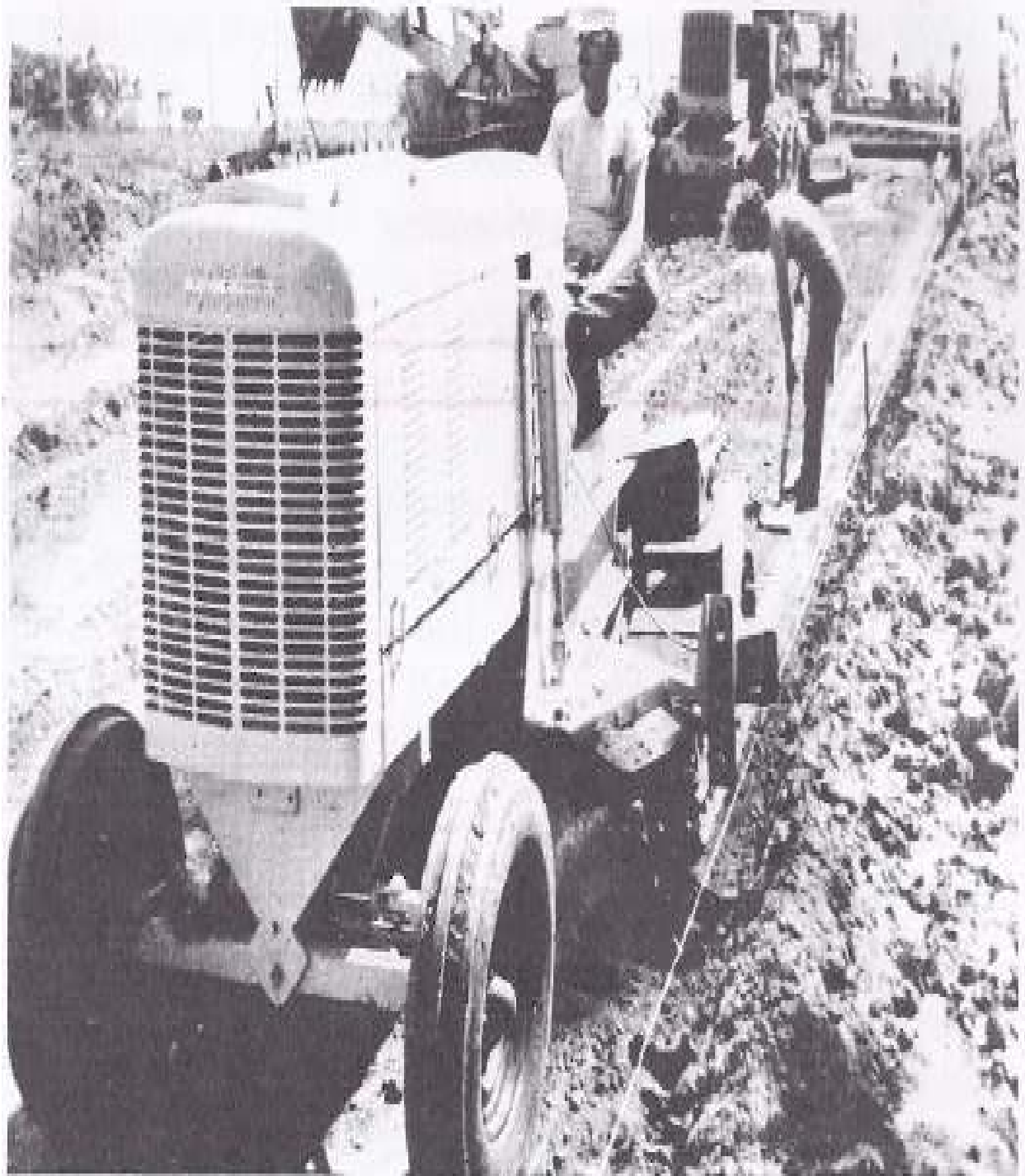
FIGURE 20-12 Cutting of trench to exact line and grade, prior to placing of forms. (Courtesy Portland Cement Association.)
