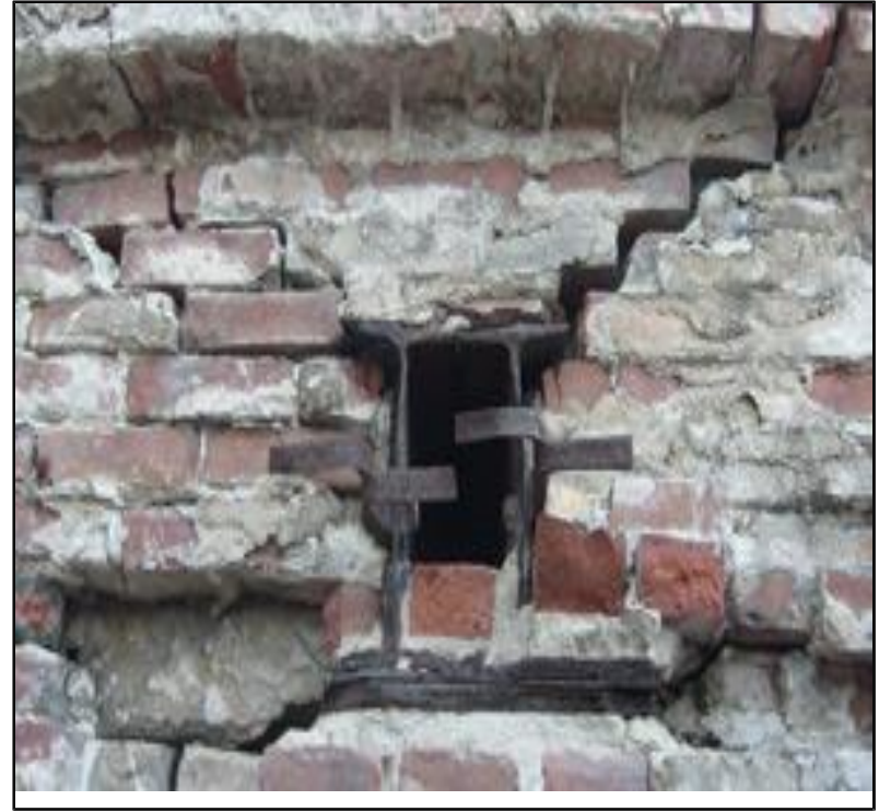
Corrosion of embedded steel
