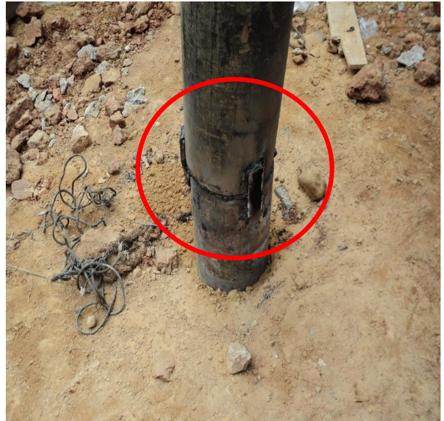
A joint of king post became weaker
