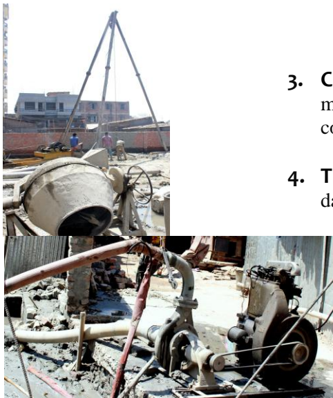
Figure 4: Casting machine on pit
