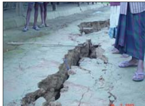
2003: Long crack along River, Kolabunia
