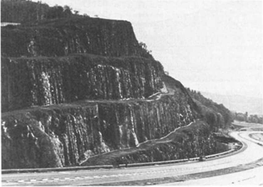
Figure 7.13 Pre-split rock surface in a road cutting for the M90 motorway near Perth, Scotland.
