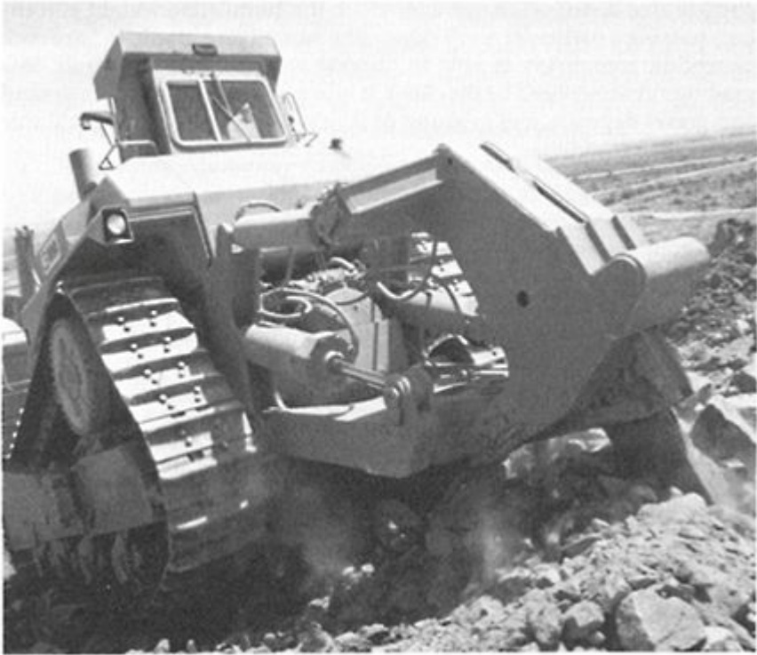
Figure 7.5 Excavation of rocks using a mechanical ripper. (Photograph by courtesy of the Caterpillar Tractor Company, Illinois.)
