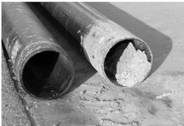
Figure 12.1: Backfill sand contaminating a new pipe at a water main construction site
