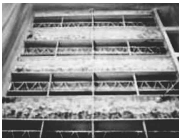
Figure 6.17: Mud balls on filter surface
