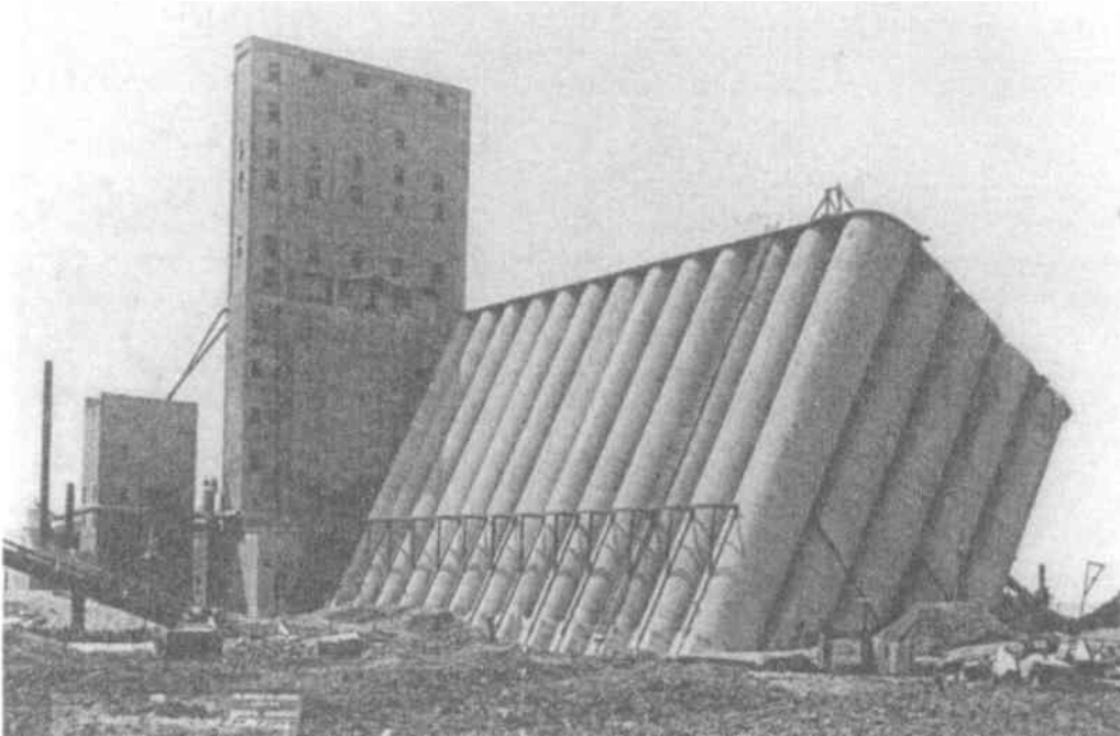
Figure 12.22 The tilted Transcona grain elevator (Courtesy: UMA Engineering Ltd., Manitoba, Canada)
