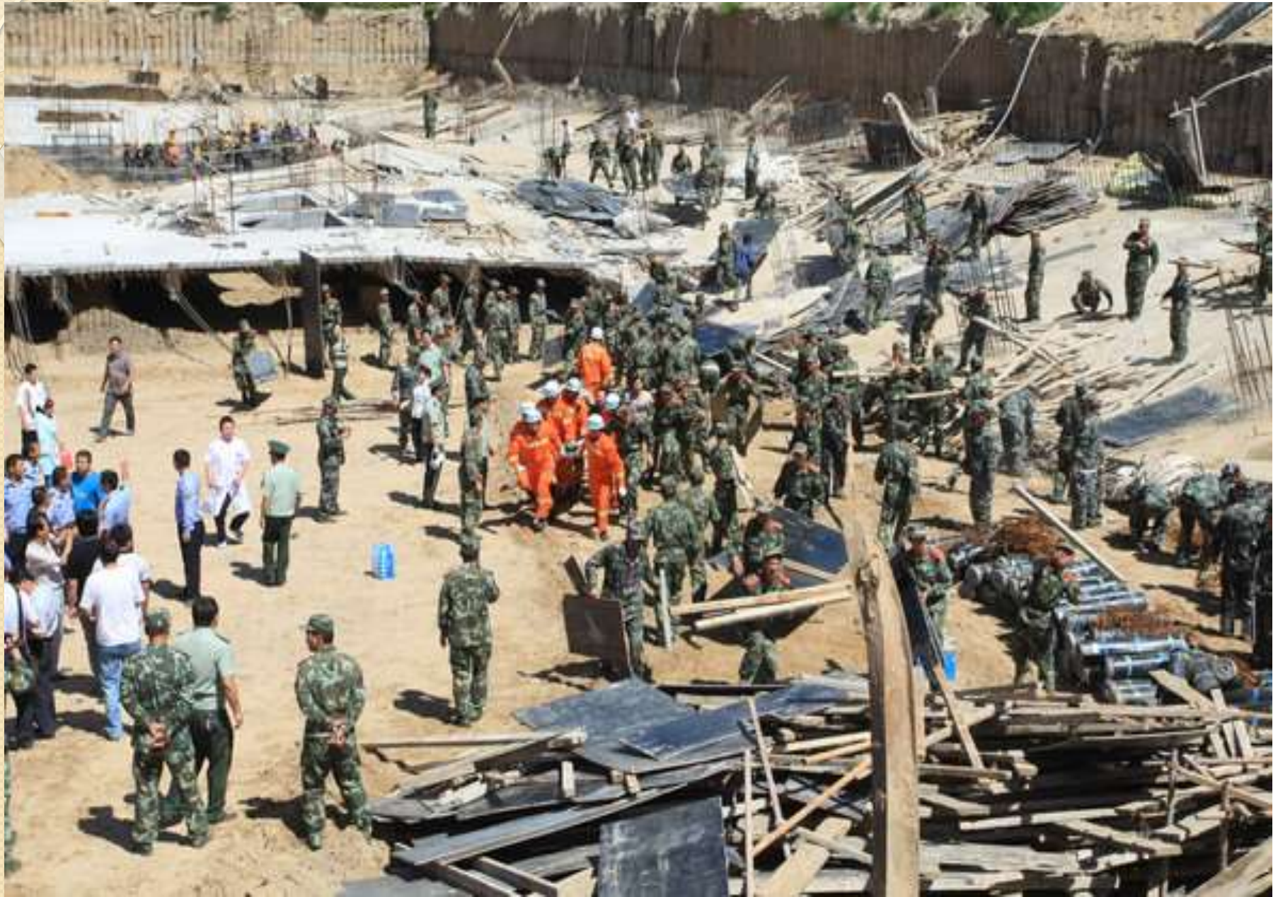
Accident during Building Construction
