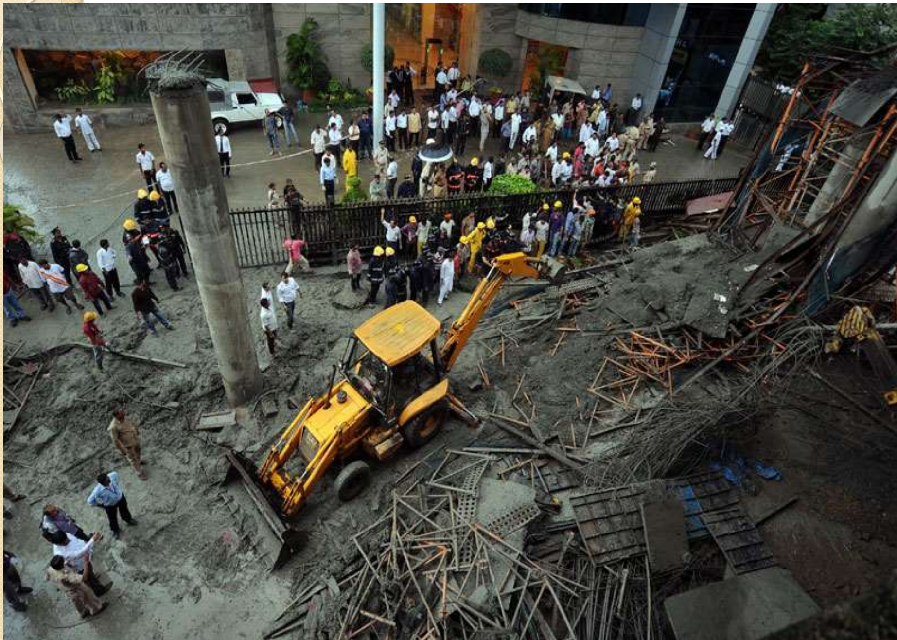
Accident during Pile Construction
