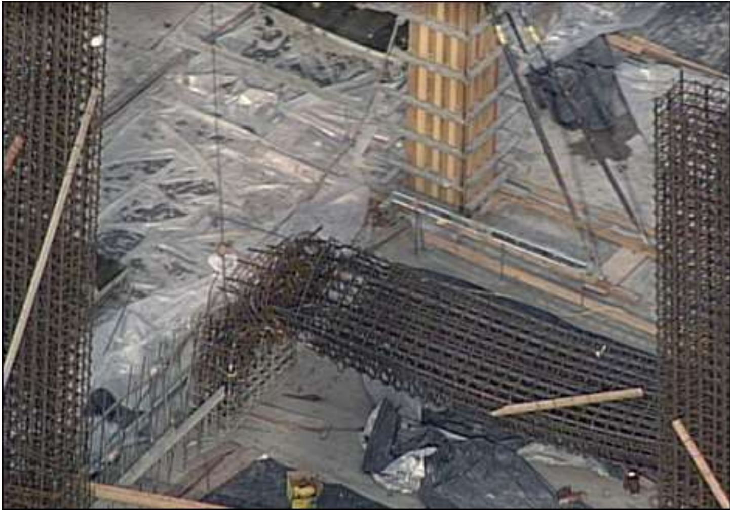
Accident during Column construction
