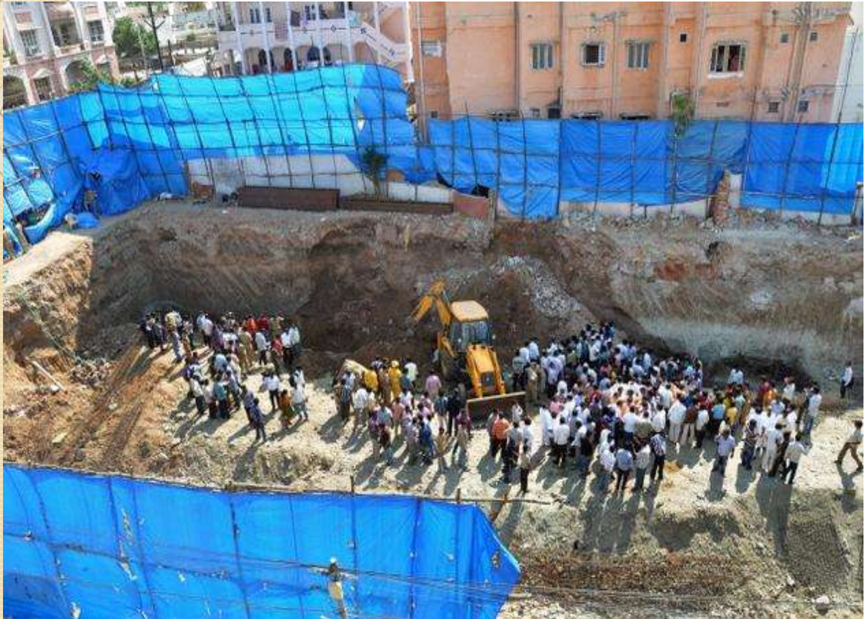
Accident during Excavation
