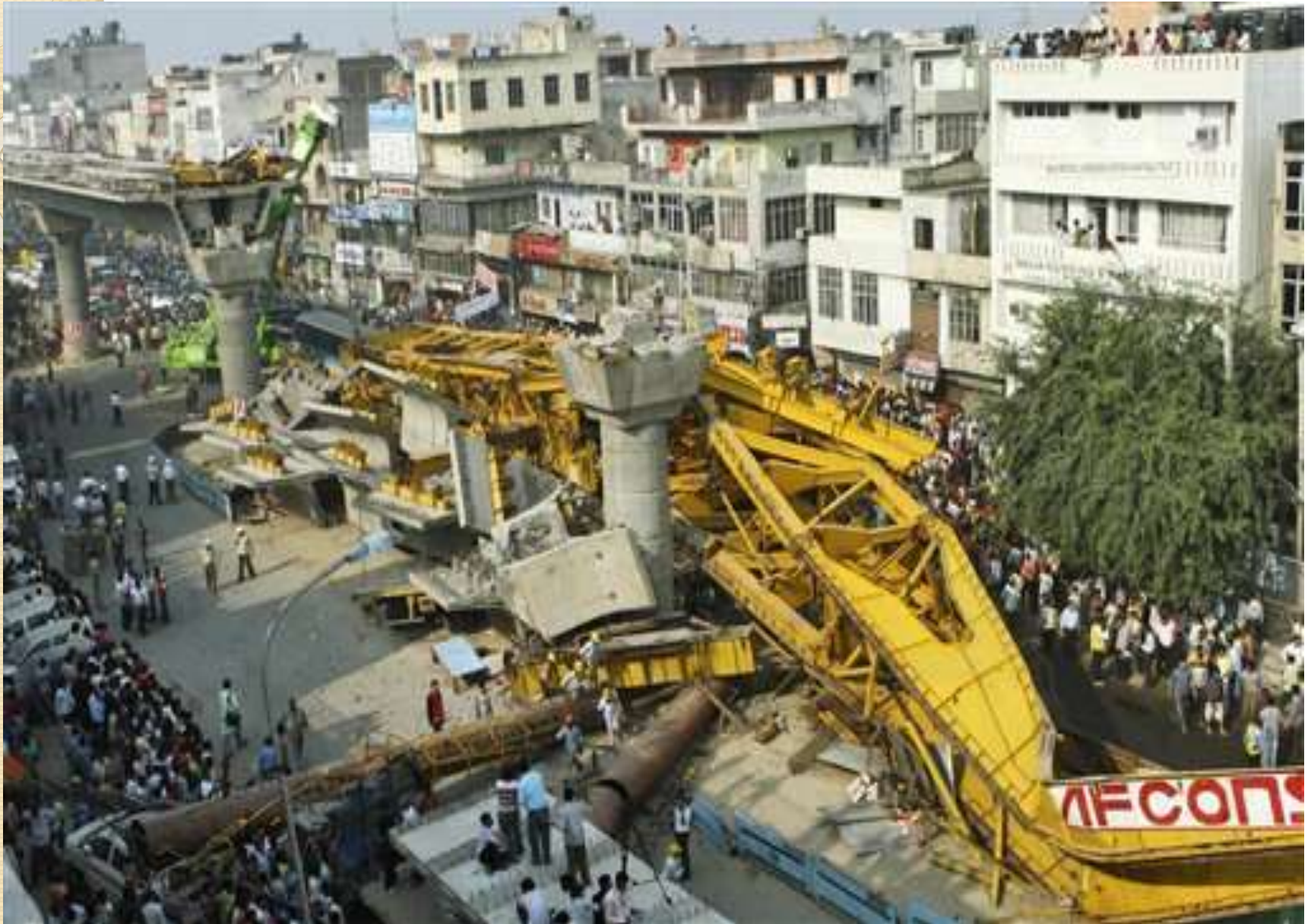
Accident during Over bridge Construction
