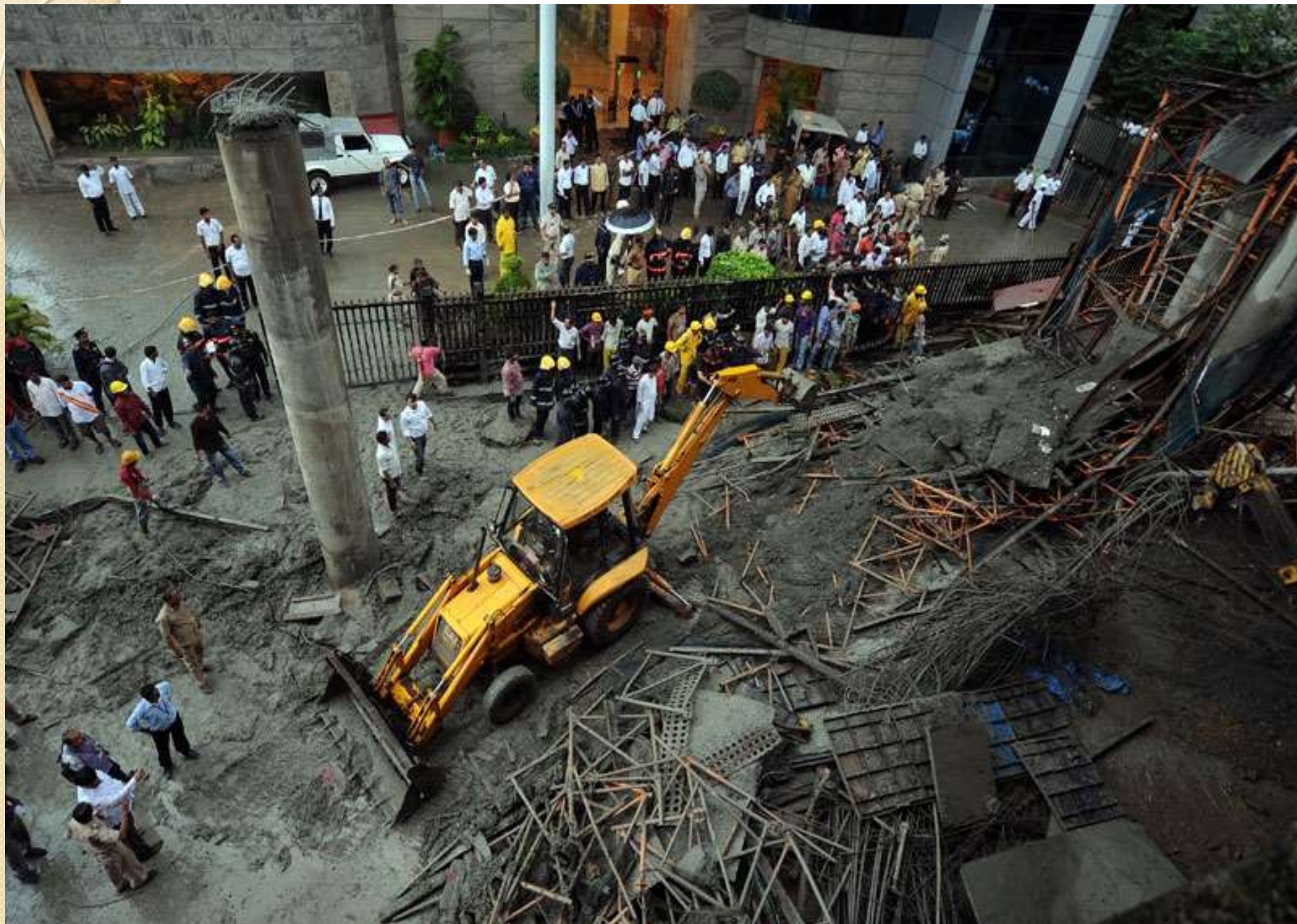
Accident during Pile Construction
