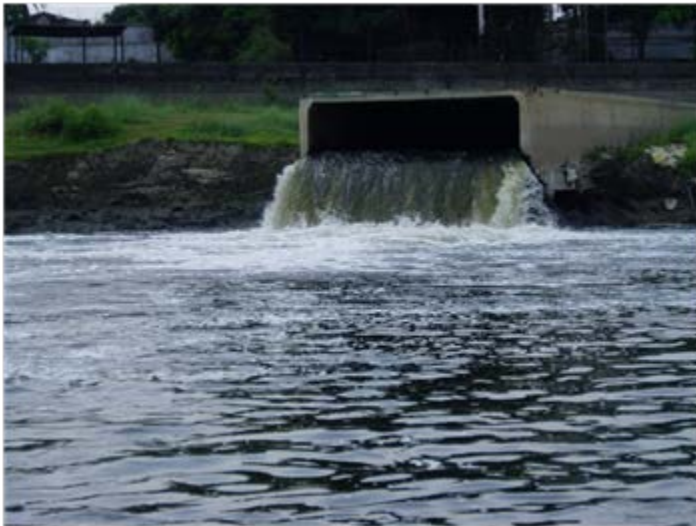
Discharge outlet of Siddhirganj 210 MW Power plant
