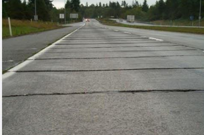
Figure 1: Faulting - looking in the opposite direction of traffic flow.
