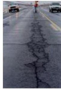
Fatigue failure from stripping
