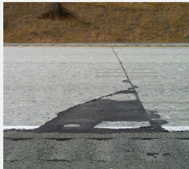
Figure 2: Patch over an area of dowel bar failure.
