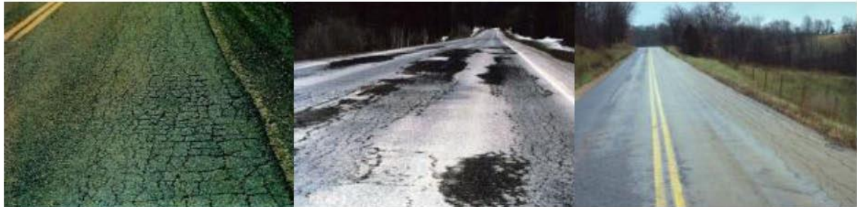
Bad fatigue cracking
