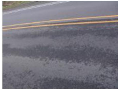
Water bleeding up close
