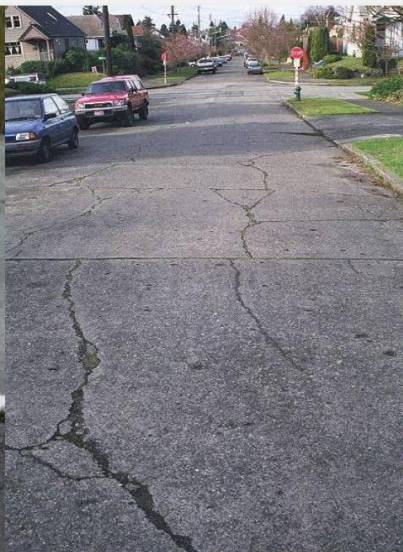
Figure 2: Multiple panel cracks on a residential street.
