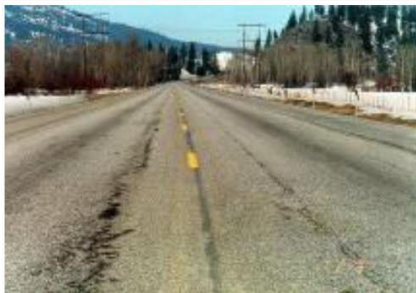
Raveling due to low density
