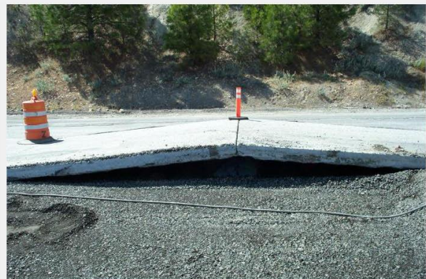
Figure 2: Blowup on SR 195 in eastern Washington.
