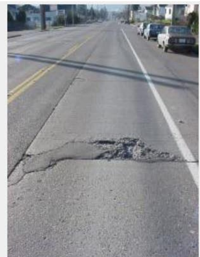
Figure 3: Bad construction joint spalling.
