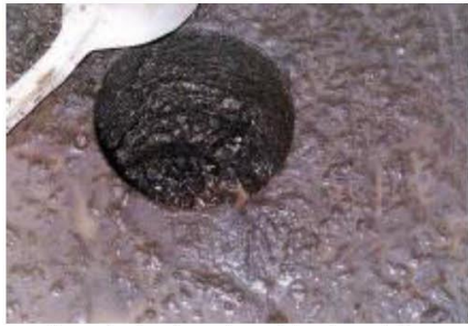
Core hole showing stripping at the bottom
