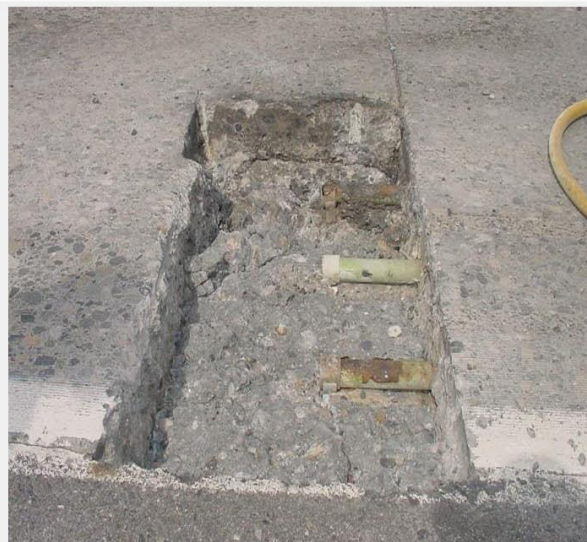
Figure 1: Dowel bar corrosion.
