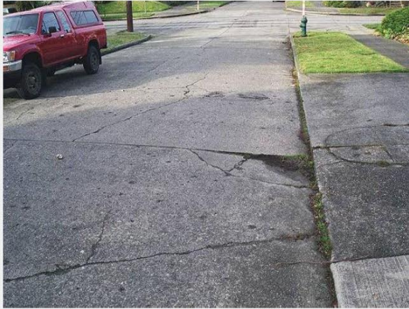
Figure 1: Corner break in Seattle, WA on a local road.
