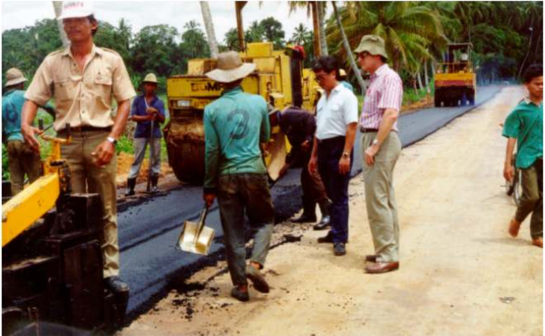
Photo 7. Asphalt Compacted immediately by Steel Wheeled Roller, with Multi Tyre Roller in distance.
