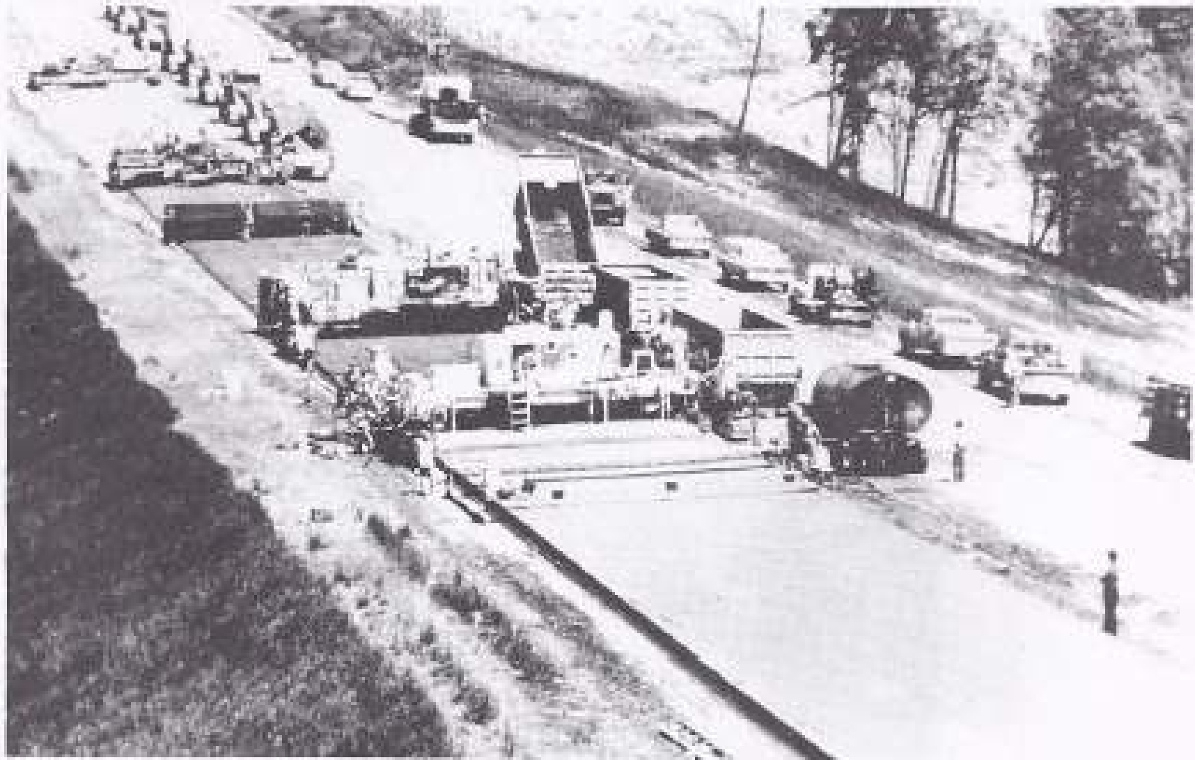
FIGURE 20-17 Slipform paver at work on an interstate project. (Courtesy Portland Cement Association.)
