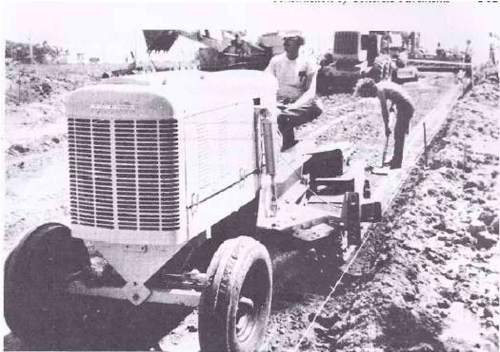
FIGURE 20-12 Cutting of trench to exact line and grade, prior to placing of forms. (Courtesy Portland Cement Association.)
