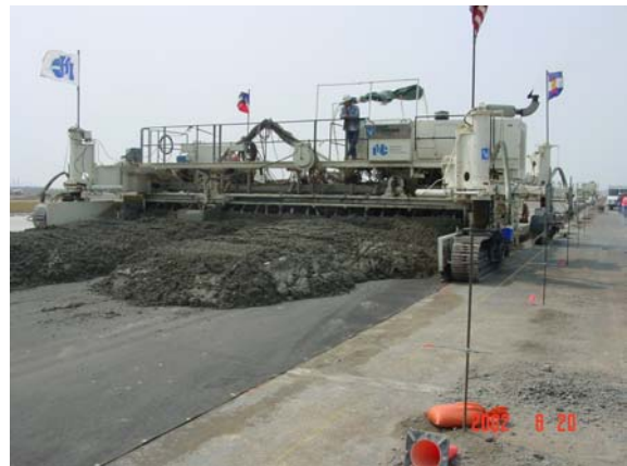
b. Maintaining uniform distribution is a good practice
