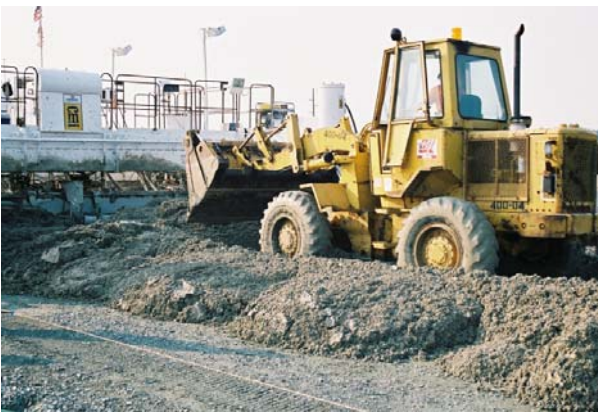
a. Use of end loader is a poor practice.
