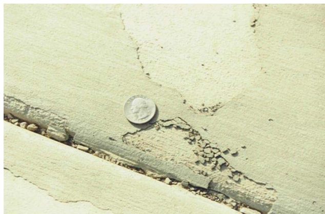
Figure 11.2 – Shallow spalling due to improper edge slump repair
