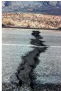
Large patched thermal crack
