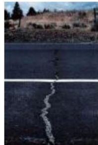
Smaller patched thermal crack
