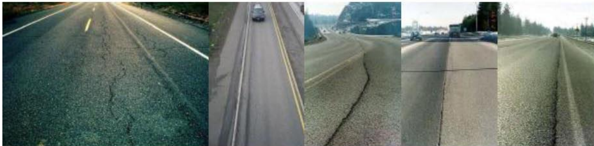
Longitudinal cracking as the onset of fatigue cracking
