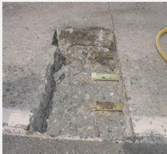
Figure 1: Dowel bar corrosion.
