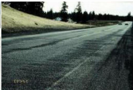
Raveling from snowplow operations
