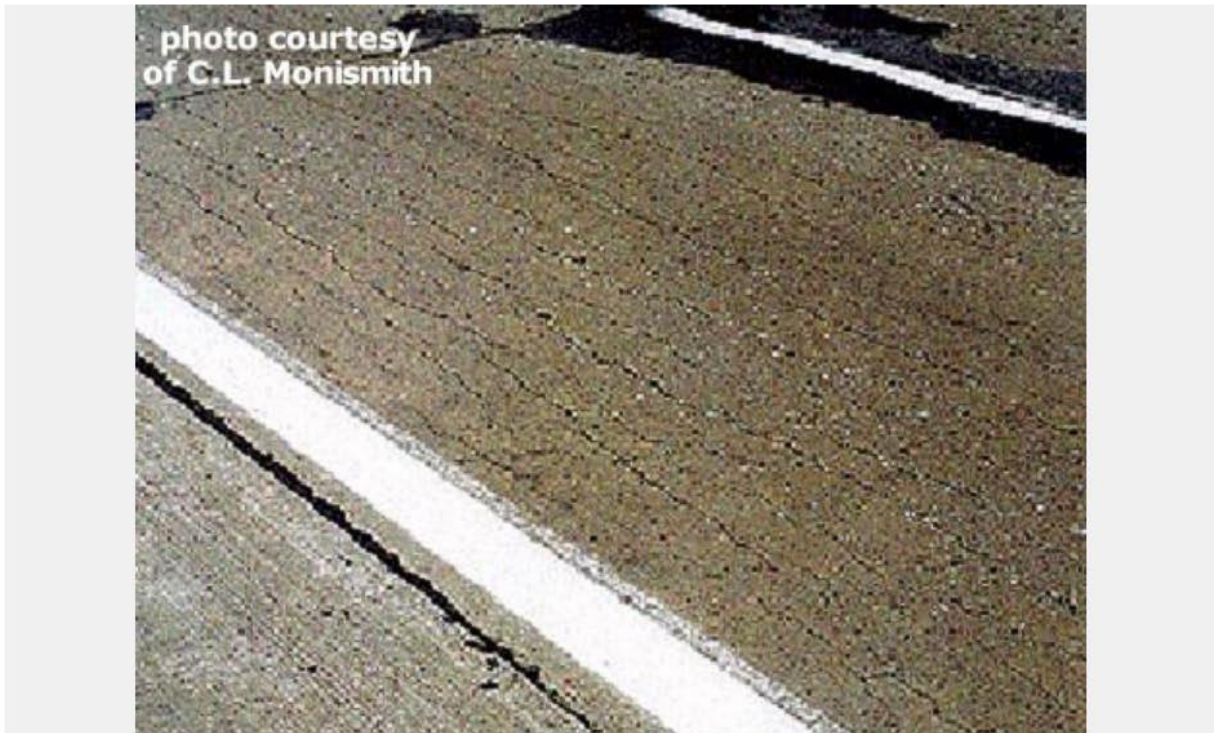
Figure 1: Severe crazing (alkali-silica reaction).
