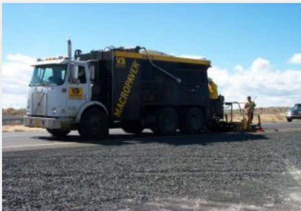
Figure 1: Ignition method major equipment.
