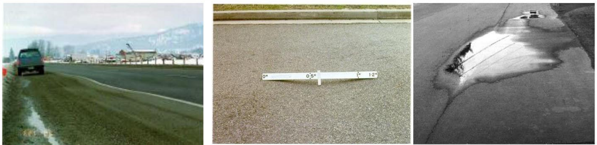
Depression in left lane and shoulder
