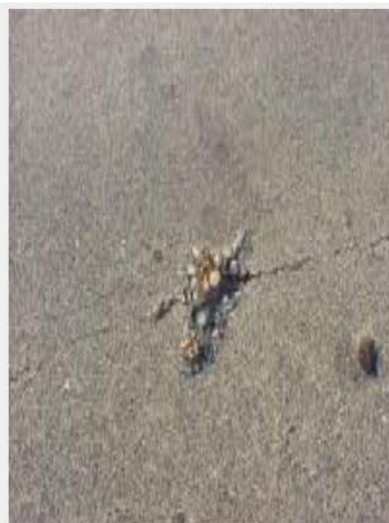
Figure 2: Onset of spalling up close.
