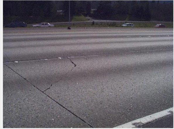
Figure 2: Corner break on a high volume road.
