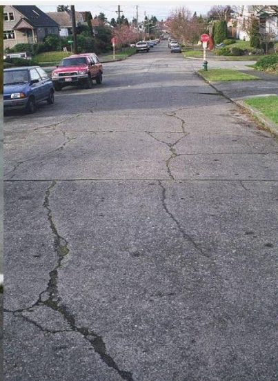
Figure 2: Multiple panel cracks on a residential street.
