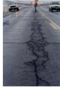
Fatigue failure from stripping
