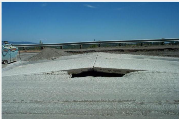
Figure 1: Blowup on SR 195 in eastern Washington.
