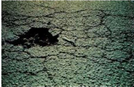
Pothole from fatigue cracking
