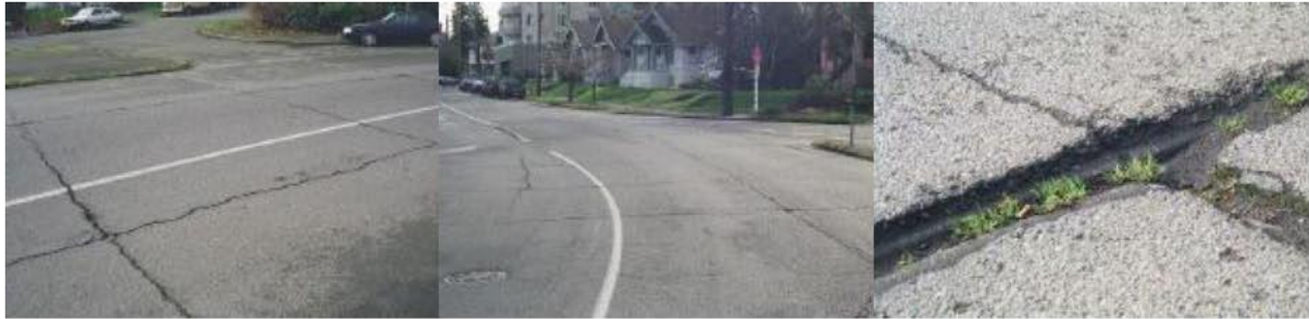
Joint reflection cracking on an arterial
