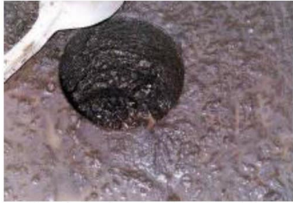
Core hole showing stripping at the bottom
