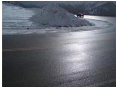
Small thermal crack
