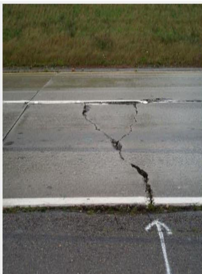
Figure 1: Large panel cracks on highway.
