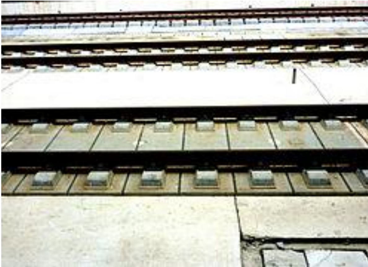
High Speed Rail, China: Ballastless tracks
