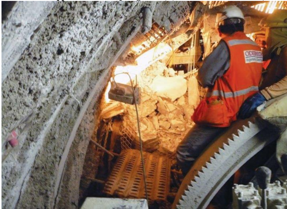
Figure.81- The 1.5km deep Olmas Trans-Andean tunnel is being cut through sever squeezing ground
