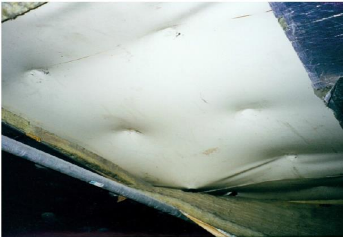
Underside of Waterproofing Membrane in Air Plenum Slab. Note that Heat Welded Attachments on the Underside of the White Membrane Receive the Insulation Panels' Anchors without Penetrating the Membrane (NCHRP, 2010)
