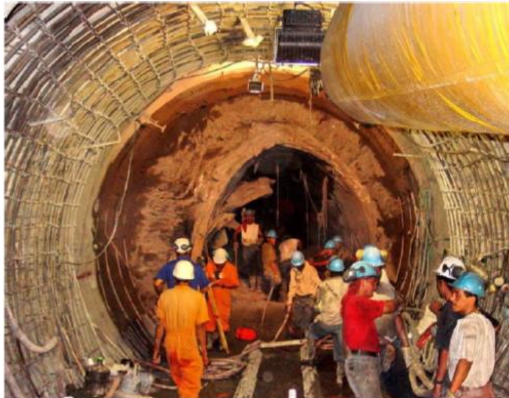
Figure.80- Failure of a tunnel section due to very severe squeezing (background) and re-mined and re-supported tunnel (foreground) (Hoek & Marinos 2009).
