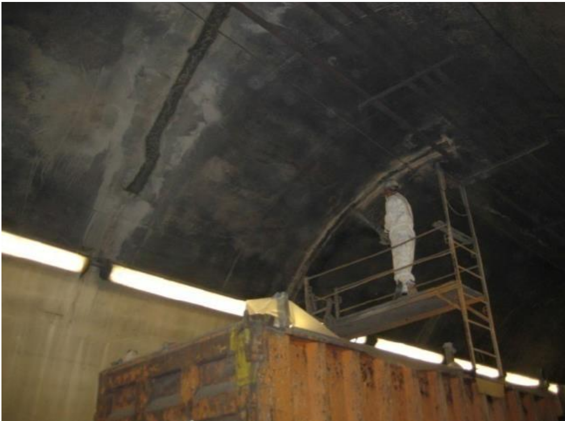
Using Shotcrete to Make Overhead Ceiling Repairs in Liberty Tunnel-Pittsburgh, PA (NCHRP, 2010)
