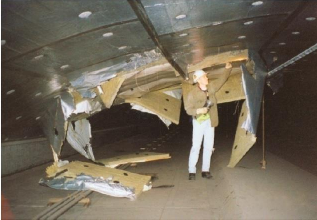
Insulated Panels under Waterproofing Membrane in Air Plenum Region above Roadway have Dislodged in an Isolated Location (NCHRP, 2010)
