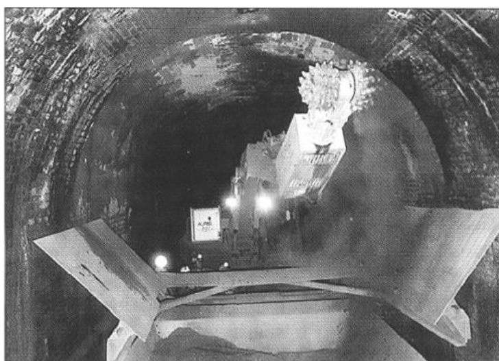
Figure.94- Laser controlled cutter for removing portions of existing tunnel liner. (Photo courtesy of Tunnels & Tunnelling North America)
