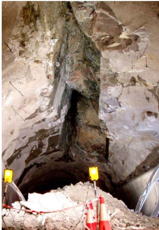
Figure .61- Image from rock fall in the Hanekleiv tunnel. The rock fall was caused by a weakness zone containing swelling clay (Picture in courtesy of Statens Vegvesen).
