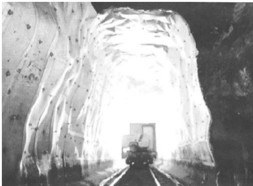
Figure.90- Insulated panels used as a waterproofing lining to keep infiltrating water from freezing. (Photo courtesy of Tunnels & Tunnelling International)
