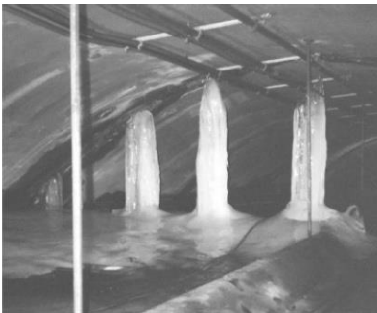
Figure.86- Ice formation at location of water infiltration in plenum area above ceiling slab
