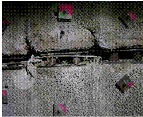
Figure 83- Yielding Support Crushed to 20 cm (One-half) (ILF, 2008)
