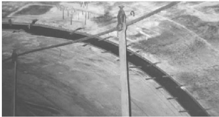
Figure.88 - Temporary drainage systems comprised of neoprene rubber troughs and 25 mm (1 in) aluminum channels.
