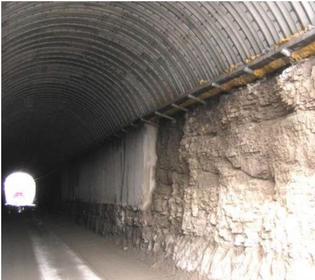
Rock Tunnel with Shotcrete Wall Repair and Arch Liner (I-75 Lima, Ohio) (2009, FHWA)
