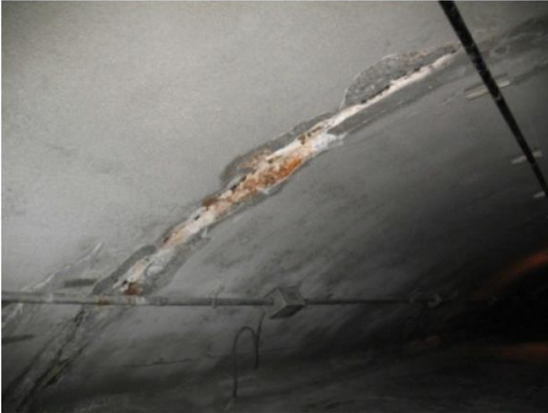
Leakage at a Construction Joint through the Cementitious Coating that was Applied on the Underside of the Tunnel Arch in a Pennsylvania Tunnel (NCHRP, 2010)
