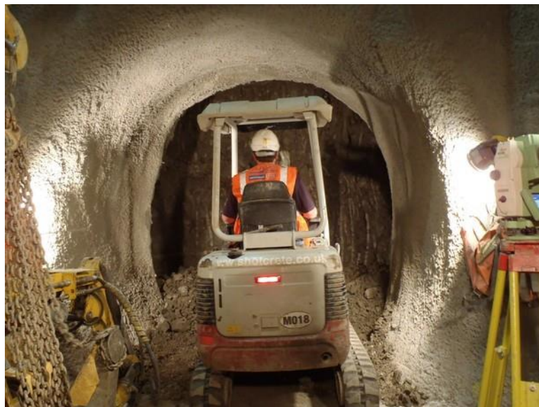
Figure.71 - The construction of Crossrail's first permanent sprayed concrete lined (SCL) tunnels on the project is now underway at Blomfield Street in the City of London.
