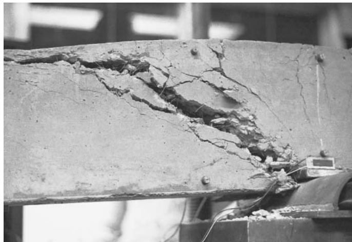
Shear failure near a middle support.
