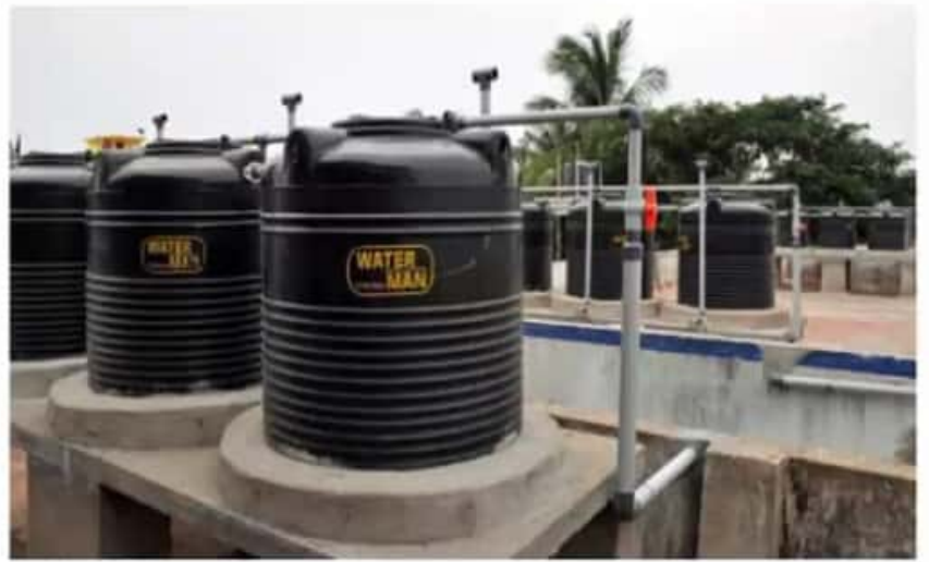
overhead water tanks
