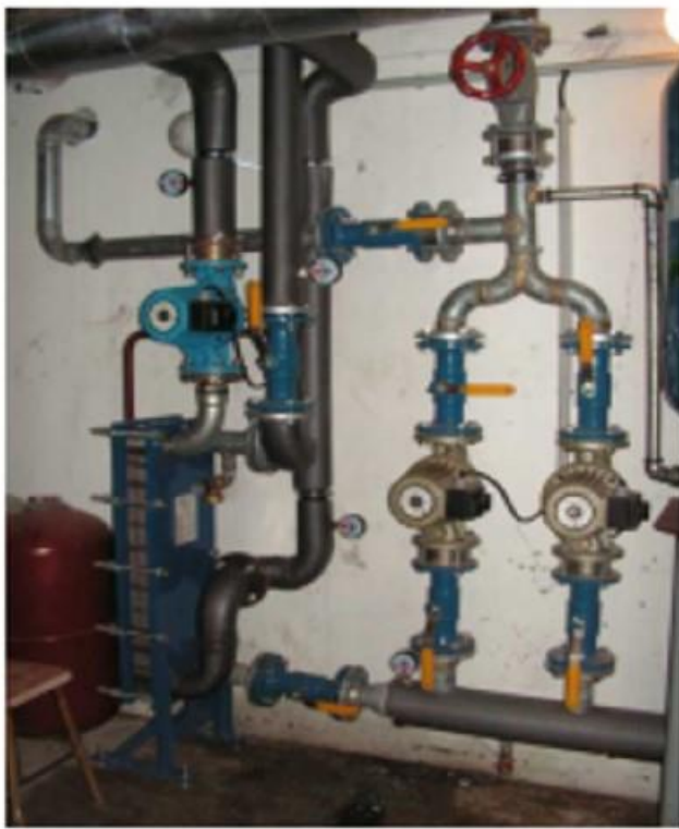
Complex pipe system
