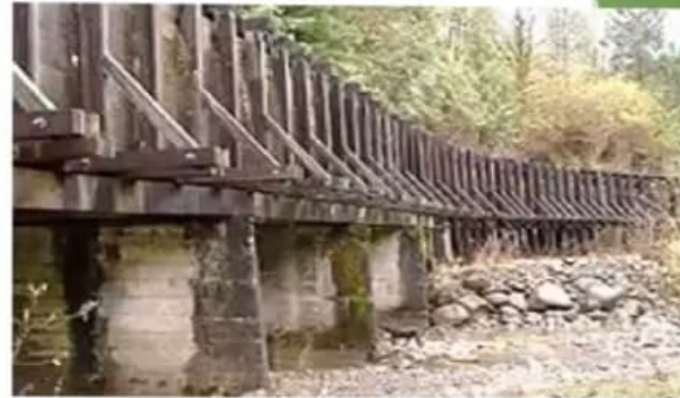
Diversion flume, carrying water from one reservoir to another.
