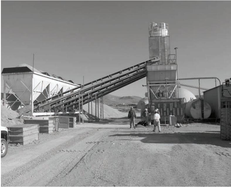
FIGURE 7.5 Concrete ready mix plant.
