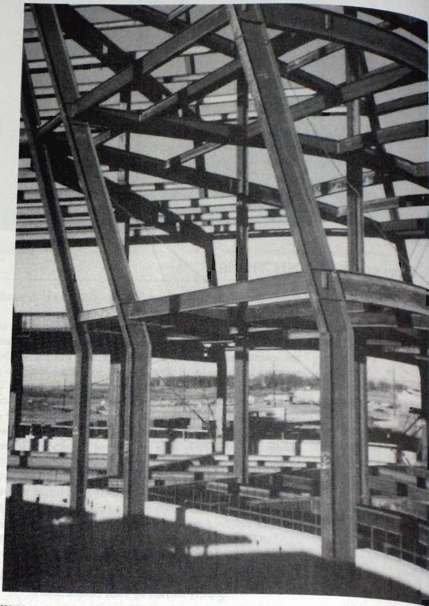
Welded connections for rigid frame construction, showing beam-to column connections with column web stiffeners. Rural Mutual Insurance Building, Madison, Wis. (Photo by C. G. Salmon)
