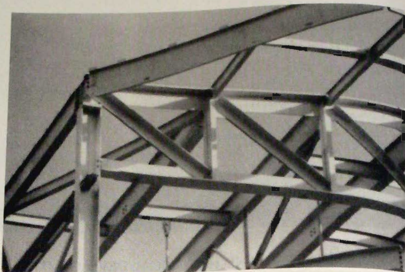
Welded truss as part of roof space truss system. (Photo by C. G. Salmon)
