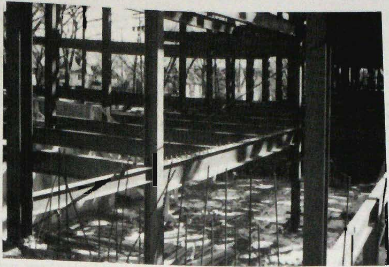
Large girder with stud shear connectors on top flange to be embedded in concrete to provide continuous lateral support (see Fig. 9.2.1b). (Photo by C. G. Salmon)
