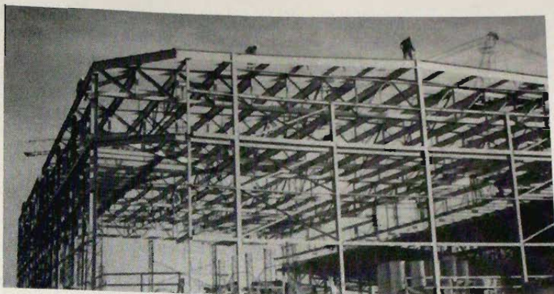
Steel framework, showing particularly the exterior columns, Southeast Recreation Facility, University of Wisconsin-Madison Campus. (Photo by C. G. Salmon)
