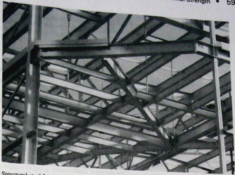
Structural steel framework at intermediate floor level. This level suspended from roof space truss with tension rods. (Photo by C. G. Salmon)
