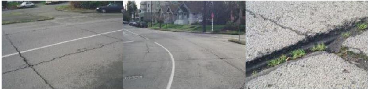
Joint reflection cracking on an arterial
