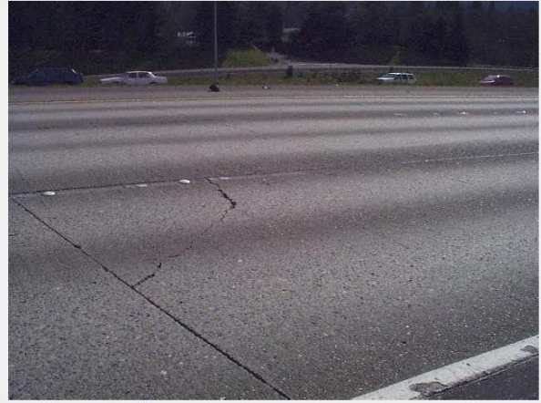
Figure 2: Corner break on a high volume road.
