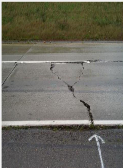
Figure 1: Large panel cracks on highway.
