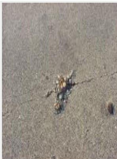
Figure 2: Onset of spalling up close.
