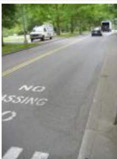
Slippage cracking at a bus stop
