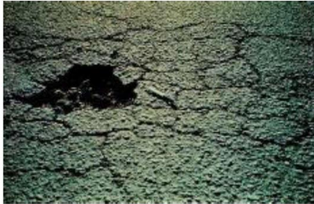
Pothole from fatigue cracking
