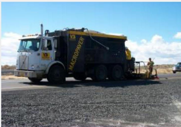
Figure 1: Ignition method major equipment.
