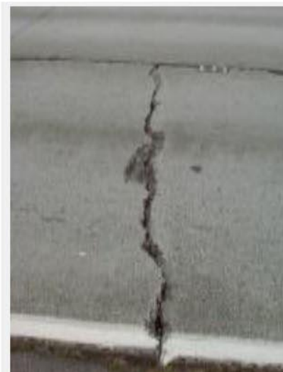
Figure 1: Spalling along a linear (panel) crack.
