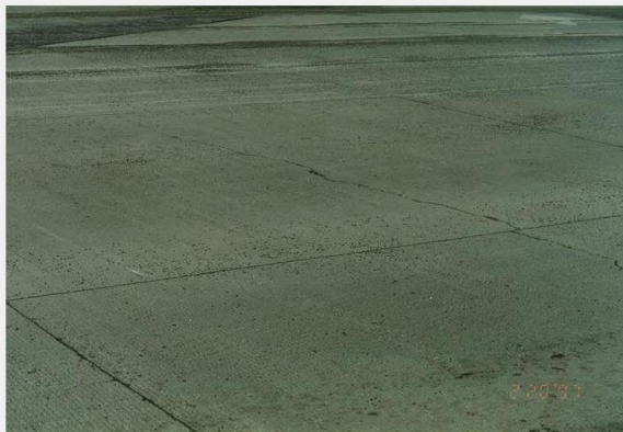
Figure 1: Shrinkage cracking on new slabs.
