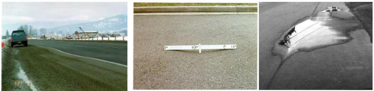
Depression in left lane and shoulder
