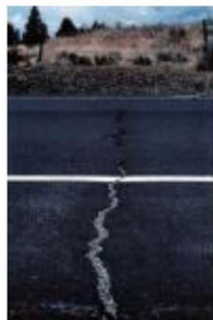
Smaller patched thermal crack
