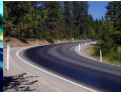
HMA bleeding from over-asphalting
