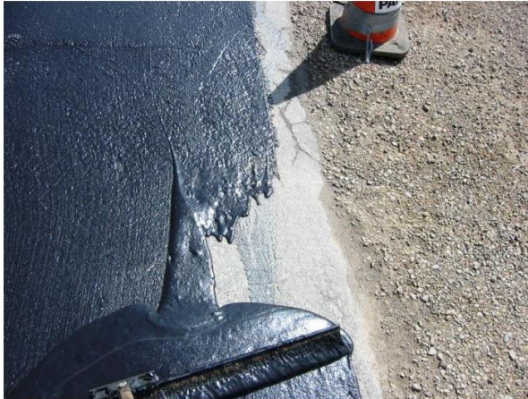
Slurry seal close-up.
