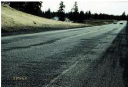
Raveling from snowplow operations
