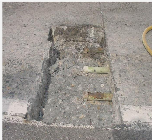
Figure 1: Dowel bar corrosion.
