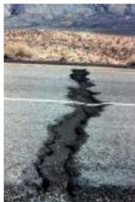
Large patched thermal crack
