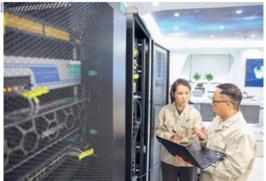
Staff members of the Electric Power Research Institute of State Grid Chongqing Electric Power Co. check equipment to protect it against cyberattacks in Chongqing Municipality on September 25
