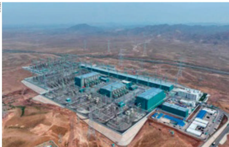
The Zhongning converter station in Zhongwei, Ningxia Hui Autonomous Region, on June 29. The station is the starting point of the Ningxia-Hunan Ultra-High Voltage Direct Current Transmission Project
